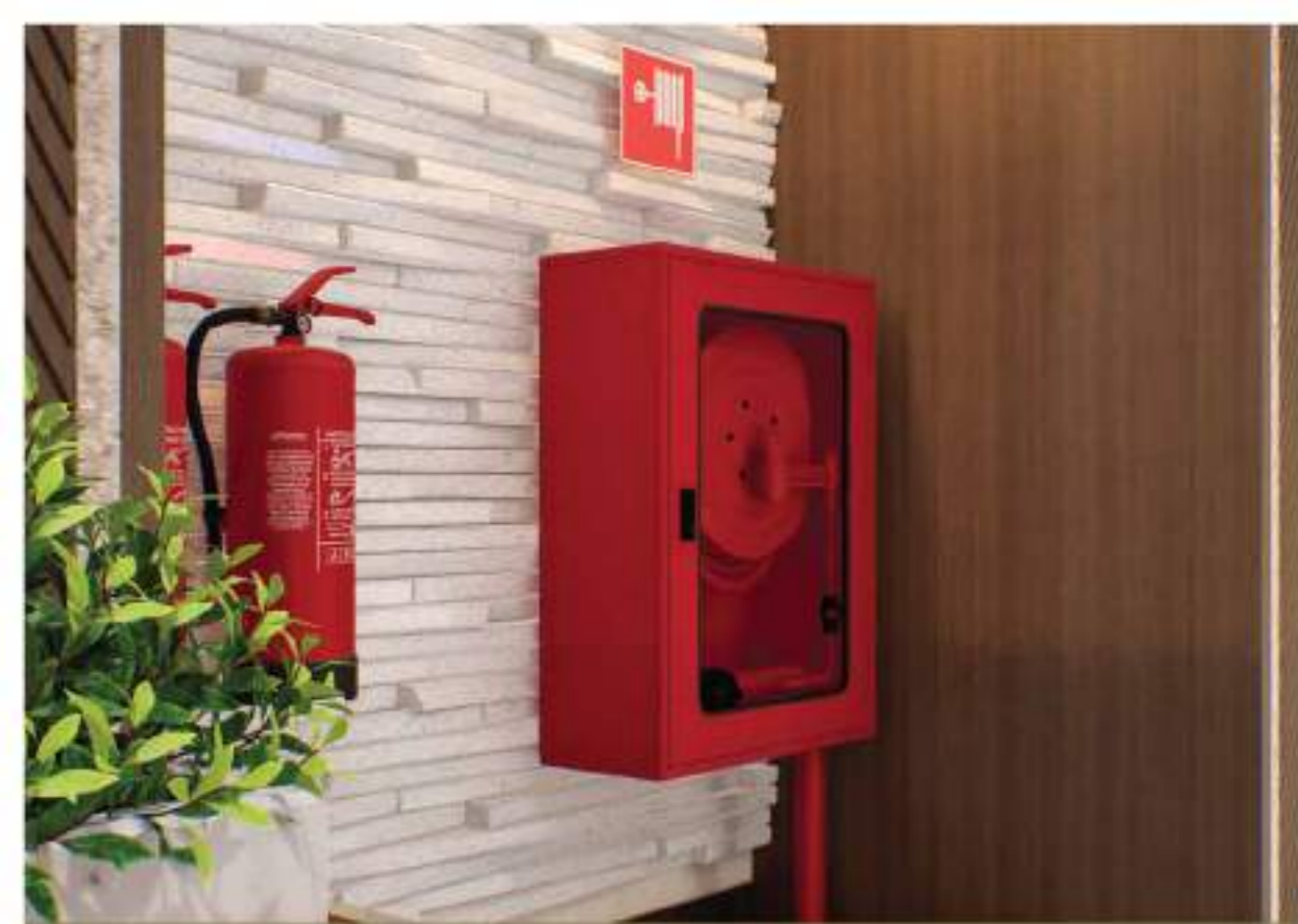
FIRE FIGHTING SYSTEM
